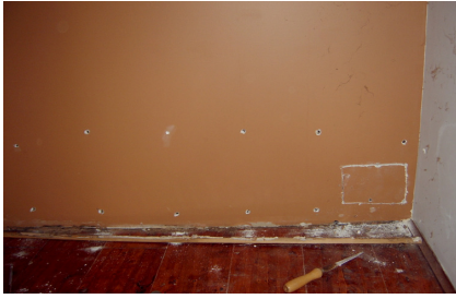
Borescope inspection to wall cavity which showed presence of termite mudding.
