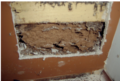
Termite mud packing to wall cavity which was discovered with the borescope & then an inspection point was cut to reveal the damaged timbers.
